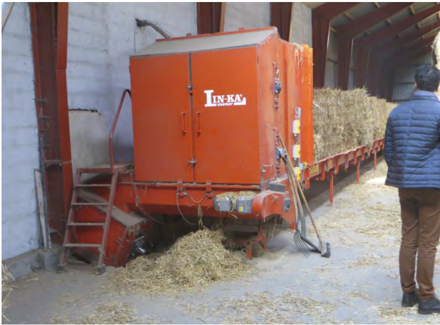
Brandstoftoevoer stro-gestookte ketels
